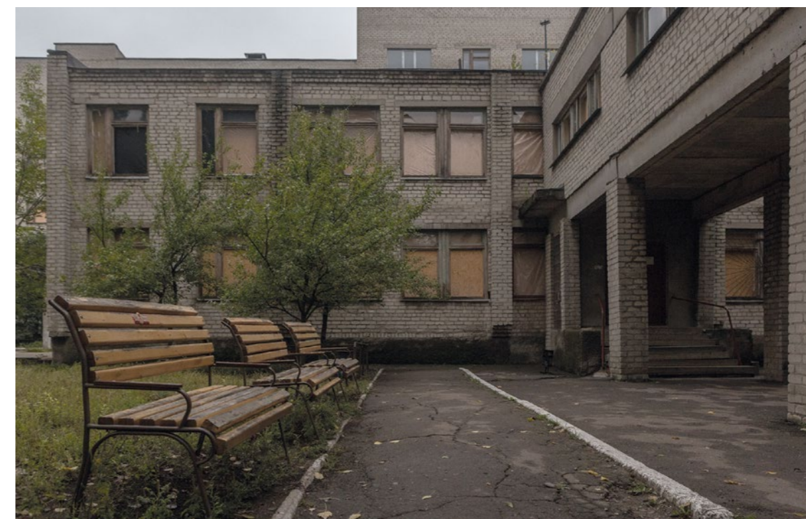
Empty benches stand outside a wing of Avdiivka City Hospital that was abandoned after two direct hits by explosive weapons. © Anton Skyba for International Human Rights Clinic at Harvard Law School and PAX / September 2016.
