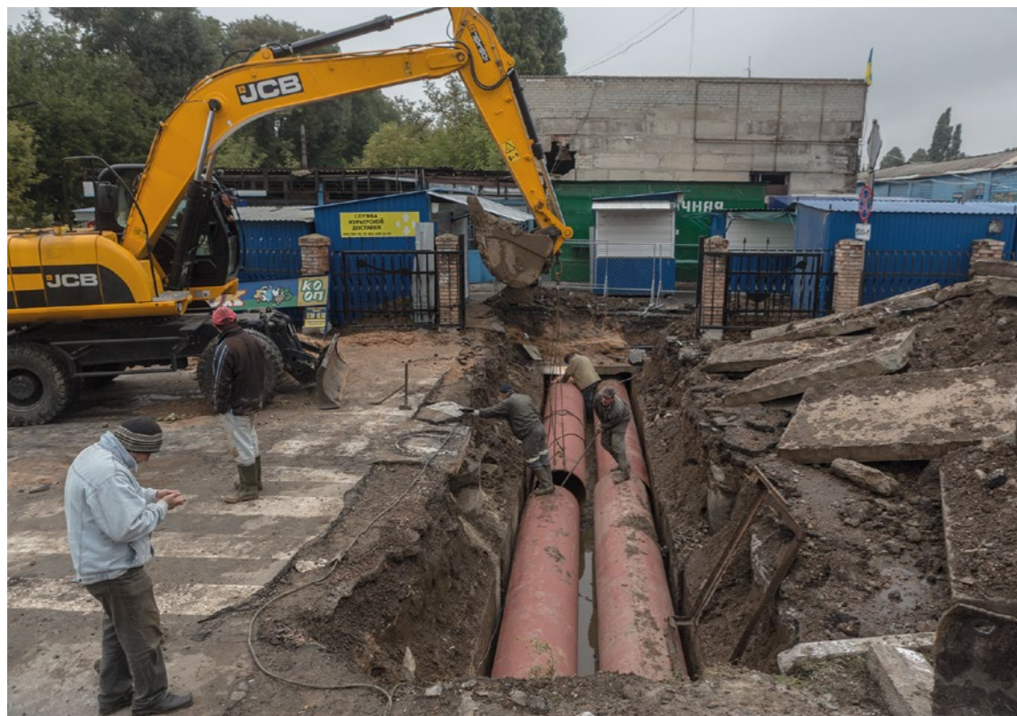
Workmen repair heating pipes near Avdiivka City Hospital in September 2016. Shelling has often presented obstacles to repairing damaged infrastructure in the east of Ukraine. © Anton Skyba for International Human Rights Clinic at Harvard Law School and PAX / September 2016.
