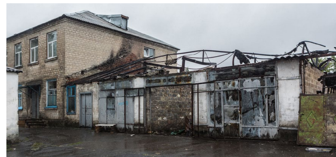
In June 2015, explosive weapons destroyed the ambulance garage of the Krasnohorivka ambulance substation and left a burned ambulance in the far right bay. Fire also damaged the adjacent neurology building of Maryinka District Central Hospital (left). © Anton Skyba for International Human Rights Clinic at Harvard Law School and PAX / September 2016.
