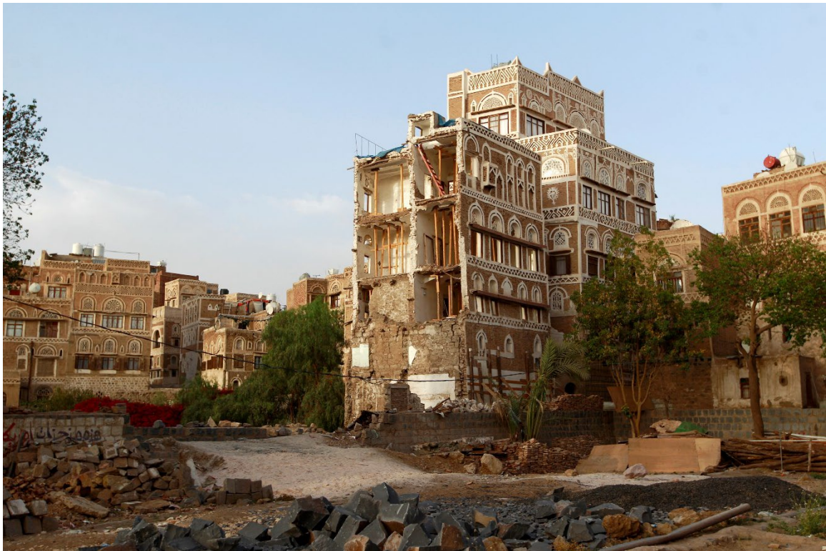
The bombing of the Old City of Sanaa by Saudi and UAE-led coalition forces in 2015 killed, injured, and displaced residents and damaged the fragile ancient building materials. The loss of cultural heritage also destroyed global and local history and a site meaningful to the community. © 2016 Mohammed Huwais/AFP via Getty Images
