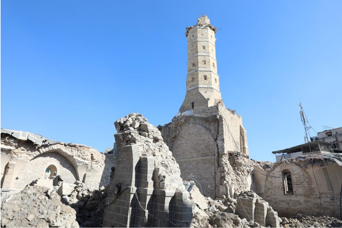
Israeli forces heavily damaged the Great Omari Mosque in Gaza through their use of explosive weapons in December 2023, leaving the courtyard full of rubble surrounded by crumbling walls. © 2024 Municipality of Gaza
