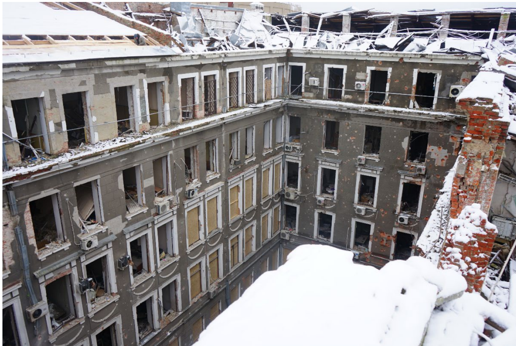
Explosive weapons used by Russian forces in March 2022 extensively damaged the roof, courtyard walls and windows, and interior rooms of the Palace of Labor in Kharkiv, Ukraine, as shown in this photograph taken in November 2022. © 2022 Viktor Dvornikov
