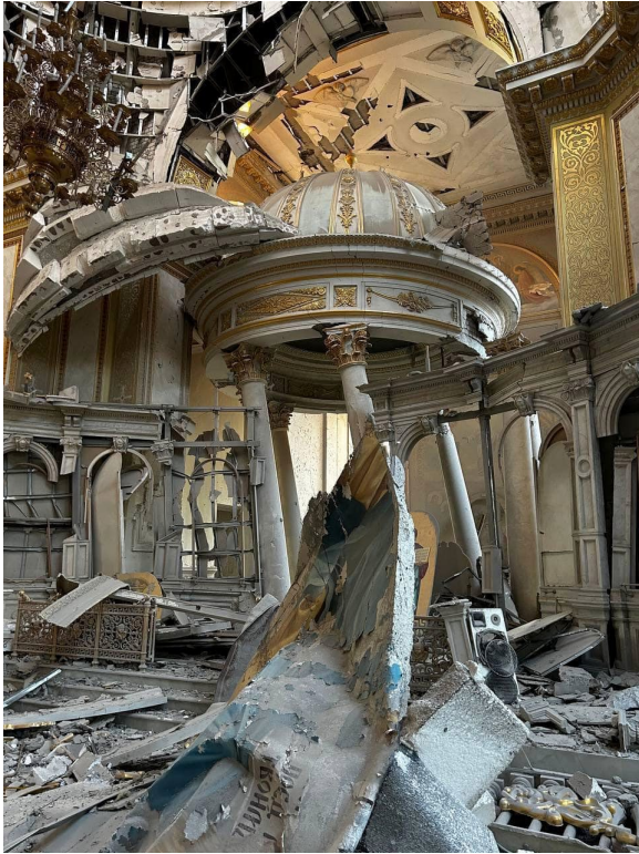
In July 2023, an explosive weapon fired by Russian forces detonated in the altar area of the Transfiguration Cathedral in Odesa. The blast and resulting fire caused walls to crumble, wall paintings and icons to burn, and parts of the roof to collapse. © 2023 Ministry of Internal Affairs of Ukraine
